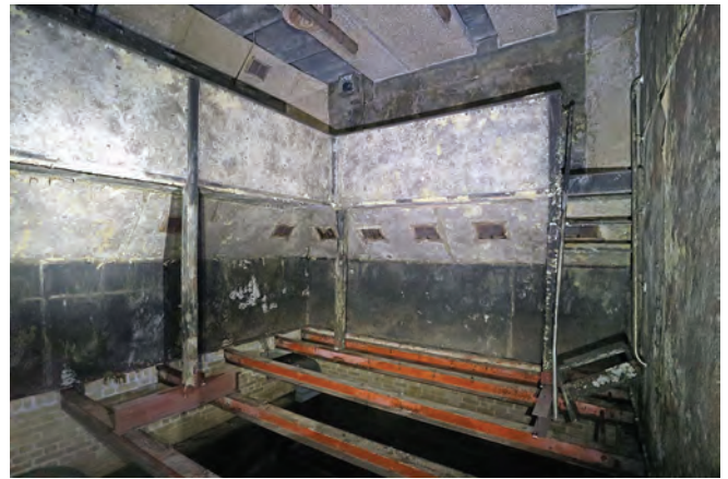
The two level Combined Filter and Plotting Room; the remains of the steps to the balcony are seen at the back of the room.
